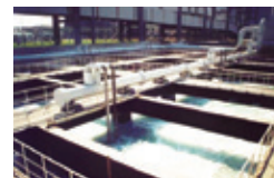
吸収廃液処理 Absorption liquid treatment system
